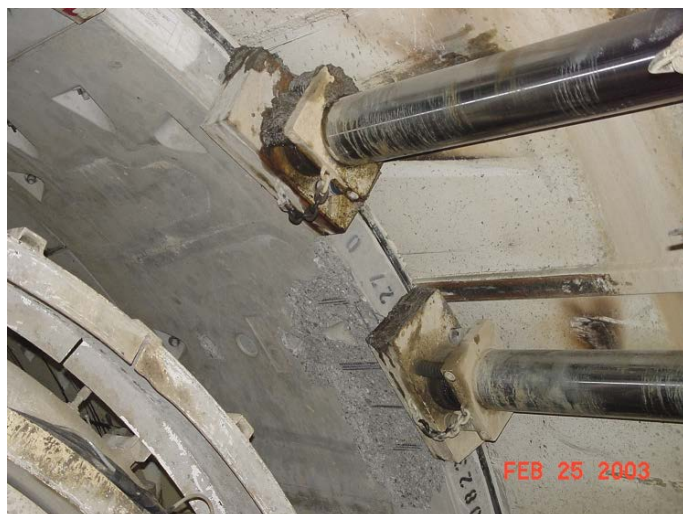
Figure 6. Edges of steel bar reinforced concrete segments breaking off when loaded by shield jacks (Herka & Schepers 2012)
