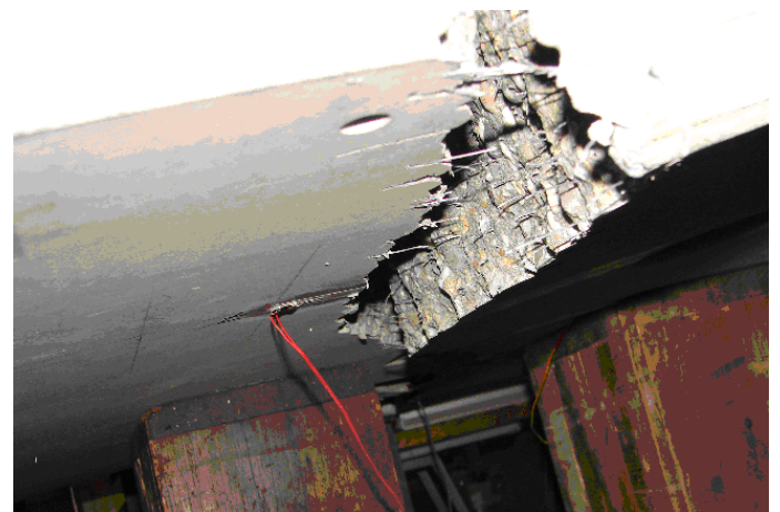
Figure 5. Steel fibres pulled out of concrete at total failure
