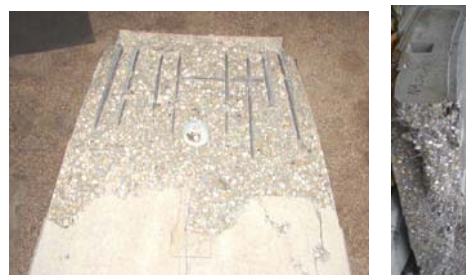
Fig. 7 Comparison of damaged key segments after reaching their capacity: a) RC key segment, b) SFRC key segment
