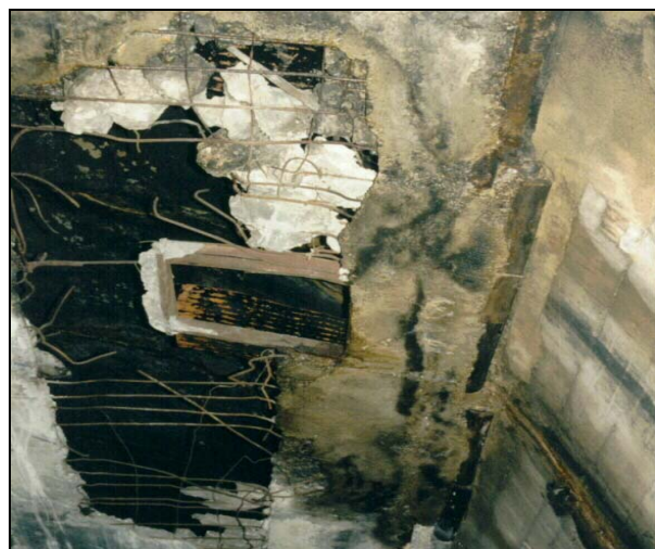
DAMAGED CEILING SLAB AT AIR OUTLET
