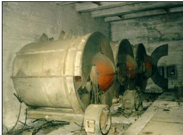
VENTILATORS AT THE SOUTH PORTAL
